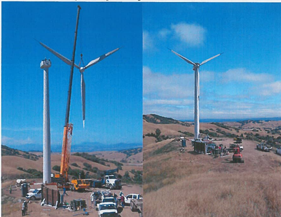
Figure 1 Example 225kW Turbine
